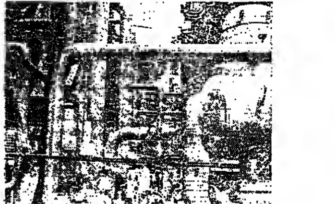
Prefabrication and erection of complete piping comprising 1,200 tonnes for fertiliser plant in India
